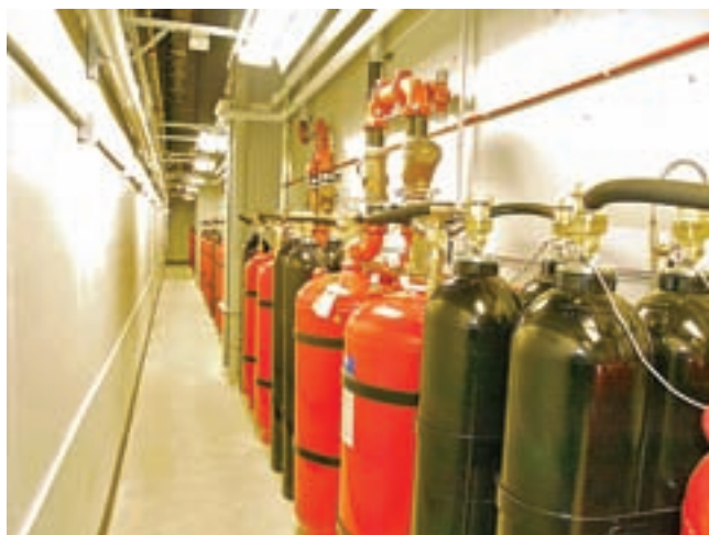
Large Clean Agent Suppression System. (Courtesy of Jeffrey Moore, P.E., Hughes Associates, Inc., Baltimore, MD)
