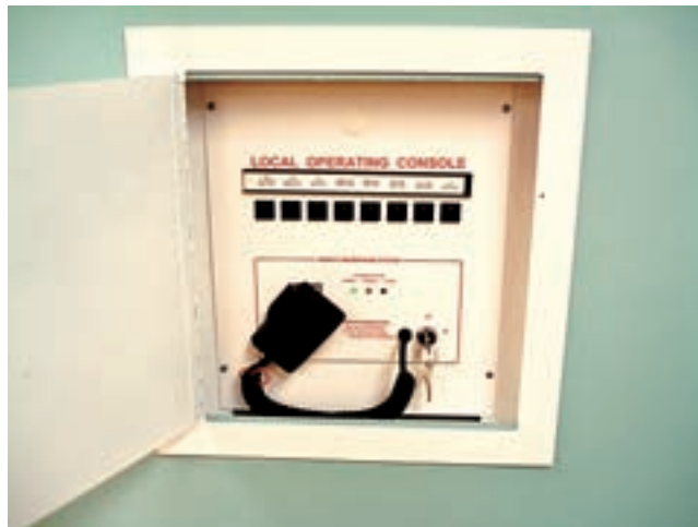
Local Operating Console. (Courtesy of Jeffrey Moore, P.E., Hughes Associates, Inc., Baltimore, MD)
