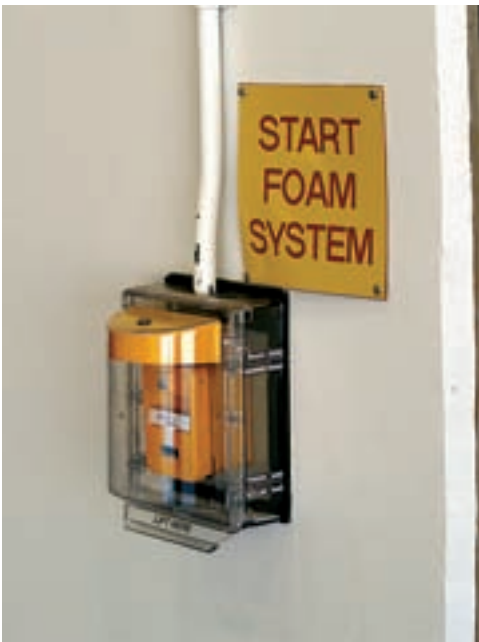
Foam Suppression Actuation Switch. (Courtesy of Jeffrey Moore, P.E., Hughes Associates, Inc., Baltimore, MD)
