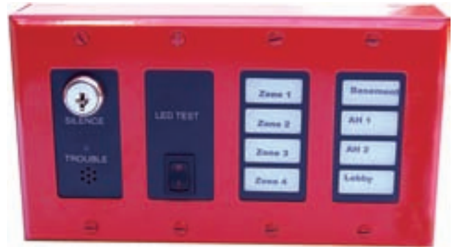
Typical Back-Lit Labeled Annunciator. (Source: Space Age Electronics, Inc., Sterling, MA)
