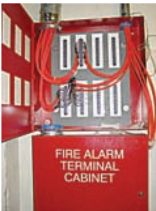
Fire Alarm Terminal Cabinet. (Source: Hughes Associates, Inc., Warwick, RI)
