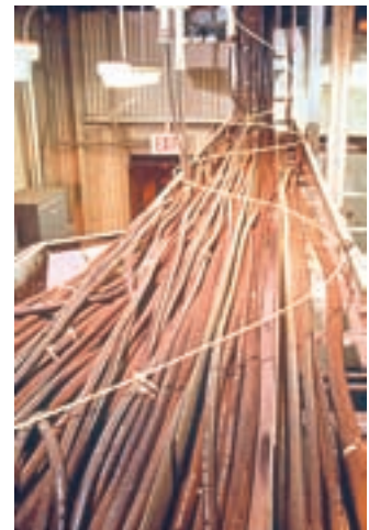
Typical Line-Type Heat Detector Installed in Cable Tray Applications. (Source: The Protectowire Co., Inc., Pembroke, MA)
