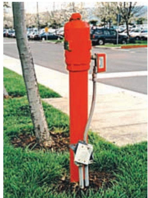
Damaged Junction Box on a Post Indicator Valve. (Courtesy of Jeffrey Moore, P.E., Hughes Associates, Inc., Baltimore, MD)
