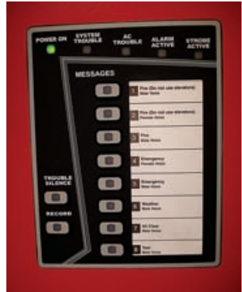
Local Operating Console with Pre- Programmed Voice Messages. (Courtesy of Jeffrey Moore, P.E., Hughes Associates, Inc., Baltimore, MD)
