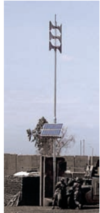
High Power Speaker Array. (Source: Cooper Wheelock, Inc. dba Cooper Notification, Long Branch, NJ)
