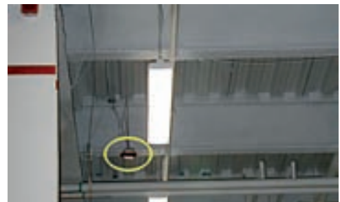
Visible Notification Appliance Suspended Below Ceiling. (Source: R. P. Schifiliti Associates, Inc., Reading, MA)
